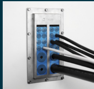
Distributor control system
